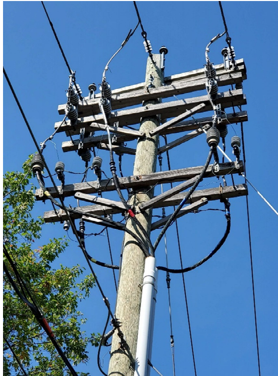
Double Circuit Riser Pole Circuits D & H
