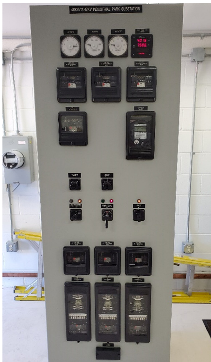
Control Panel Electro-Mechanical Relaying
