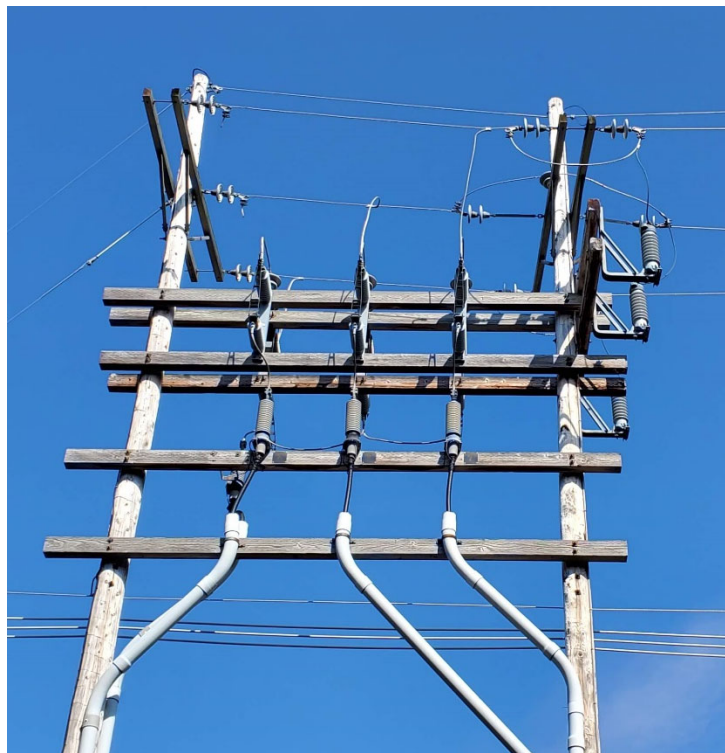
46kV Underground Cable Riser Structure
