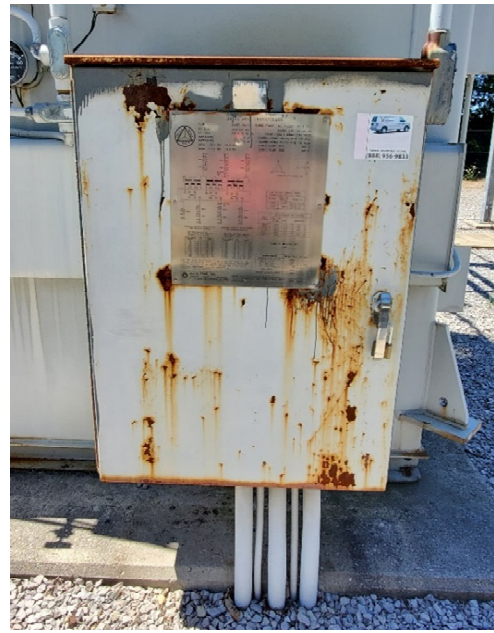
Transformer #2 – Rusting Control Cabinet
