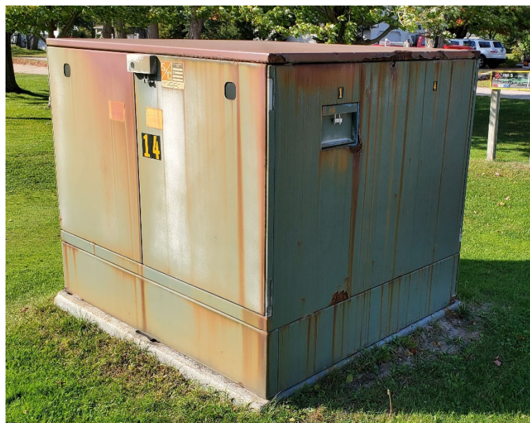
Rusting Padmount Switchgear Switch #14, Circuit I
