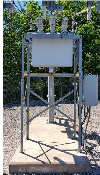
15kV Oil Circuit Recloser
