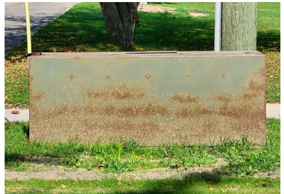
Rusting Padmount Cabinet
