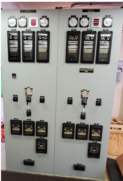
Control Panels Electro-Mechanical Relaying
