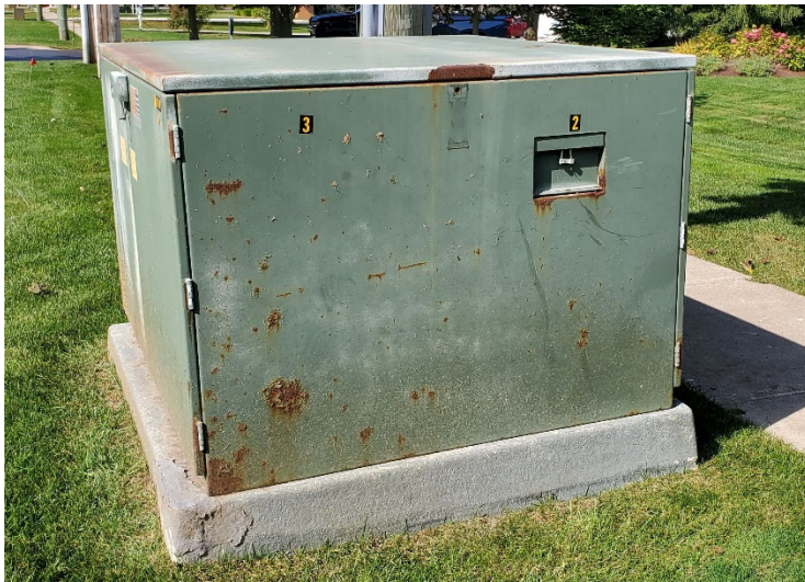
Rusting Padmount Switchgear Switch #1, Circuit E
