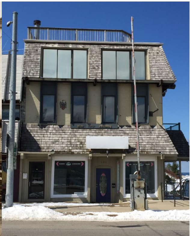
Inappropriate Replacement Windows
