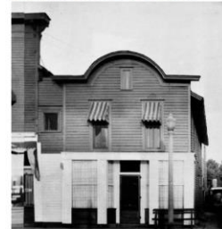
Inappropriate Storefront Modification
