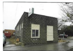
Inappropriate replacement windows
