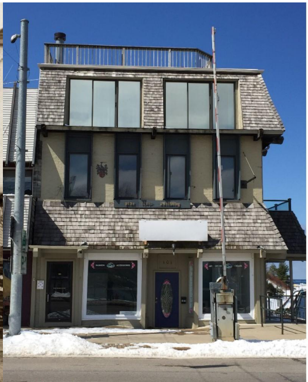
Inappropriate Replacement Windows
